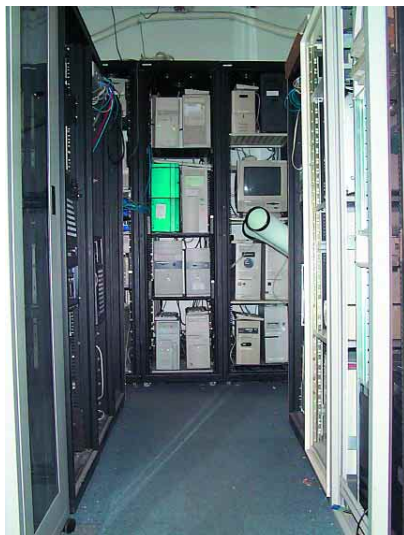
The Fulham low-cost colocation facility: a bazaar of server hardware
