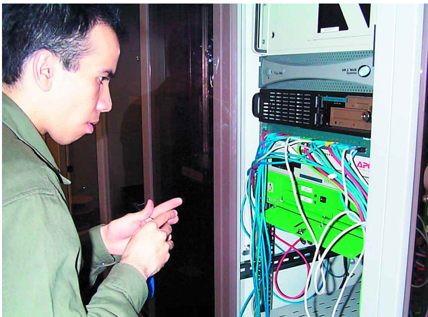
Technician Shish Batal installs a new server at Telehouse-1
