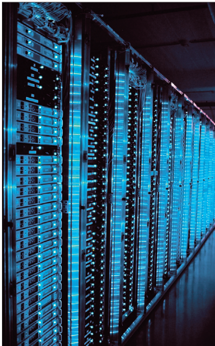
Figure 1: The 1&1 datacenter hosts around 40 percent of all domains registered in Germany – more than three million in total. Nearly all the 19” servers in a total of eleven computer rooms use Linux
