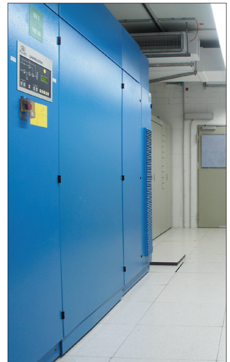
Figure 4: Each power-line is backed up by a 1.1 MVA UPS
